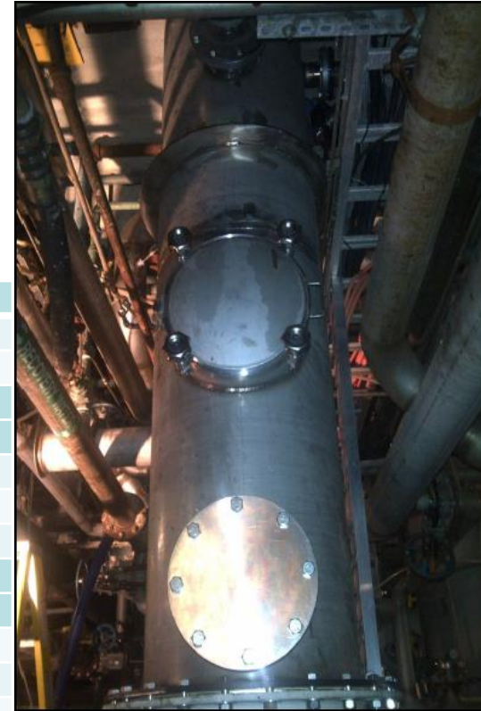
TurboScrubber® at Huhtamaki, Waterville, Maine, USA
